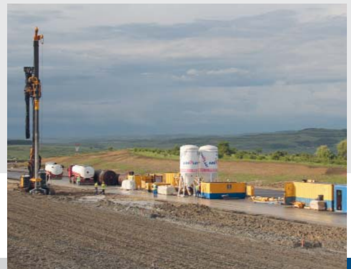
2 x MAT SCC-30 compact mixing plant, delivery pumps, agitation tank, water tank
